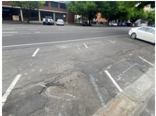
Car parking linemarking unclear Asphalt surface in poor condition
