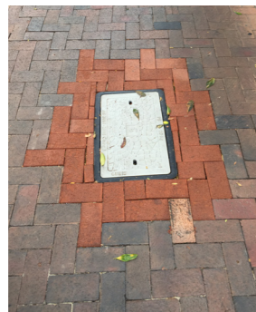
Mismatched paver reinstatements around a pit lid
