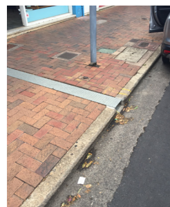
Private stormwater outlets
